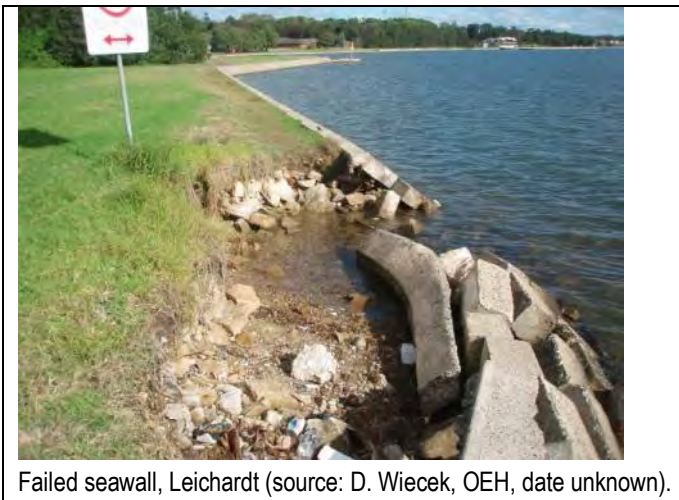
Figure 2.16: Example of Failed Seawalls
