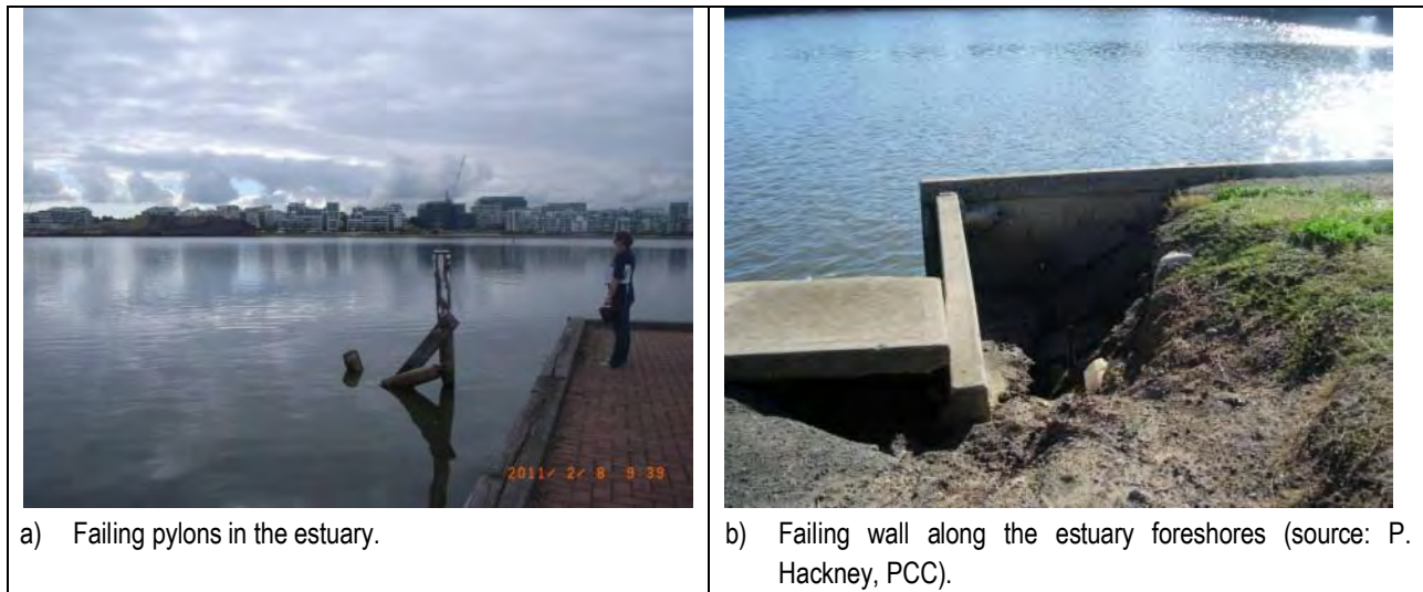
Figure 2.30: Failing Foreshore Infrastructure
