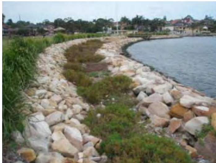
Figure 7-5: Example of an Eco-Friendly Seawall (Source: HNCMA)
