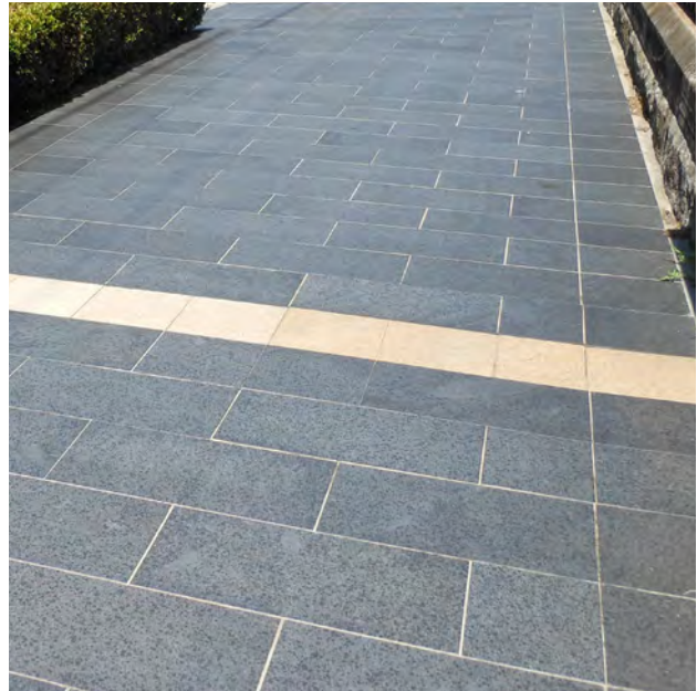
Photo 5.8. Paving Area 1. (Note: Paving Area 2 as above without the sandstone-coloured granite banding.)
