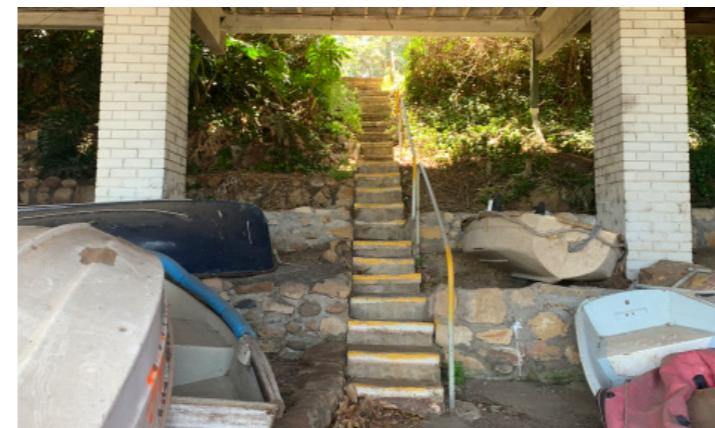
2 Non-accessible and lack of adequate lighting/security
